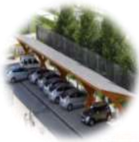
Electric vehicle charging station
