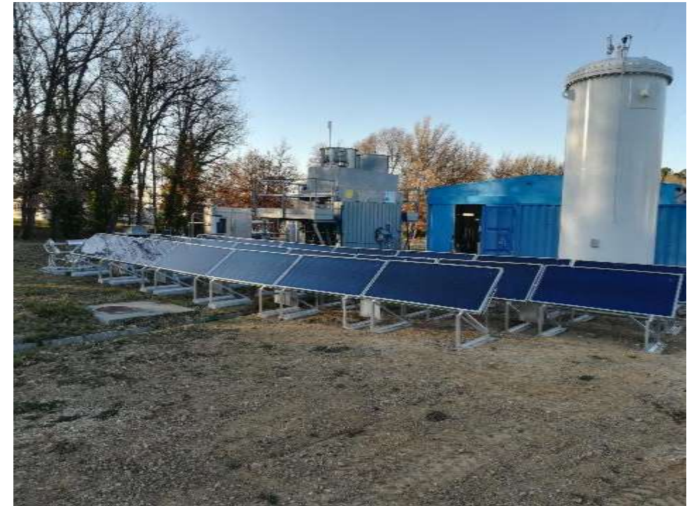
CEA Solar field
