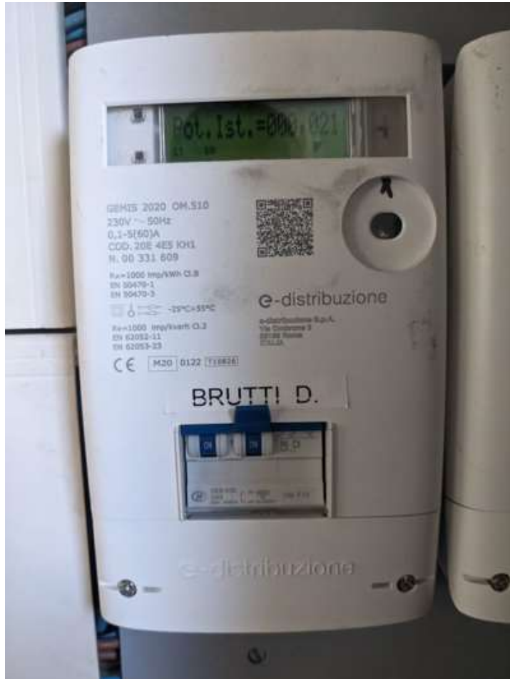
Smart meter for electricity
