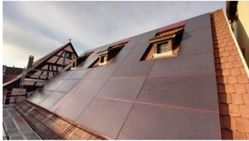
PV modules on a partially protected single family house of Bergheim (France)
