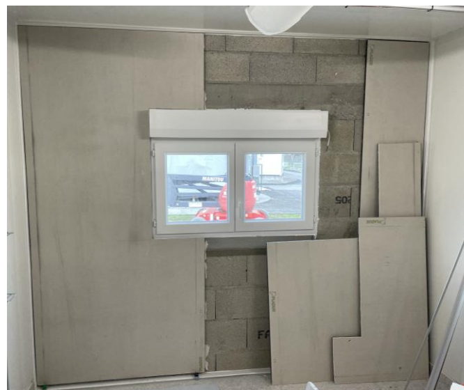
Not retrofitted façade
